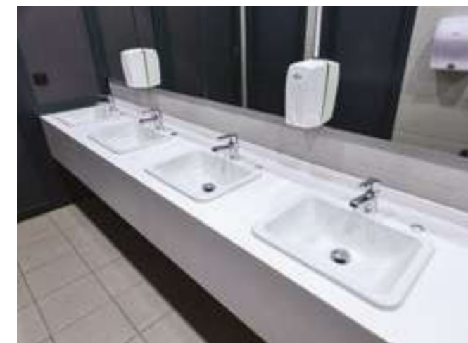
Metropole WC Pan, Arkitekta Accessories, Aquasee Basin Mixer, Loop O Control Panel
